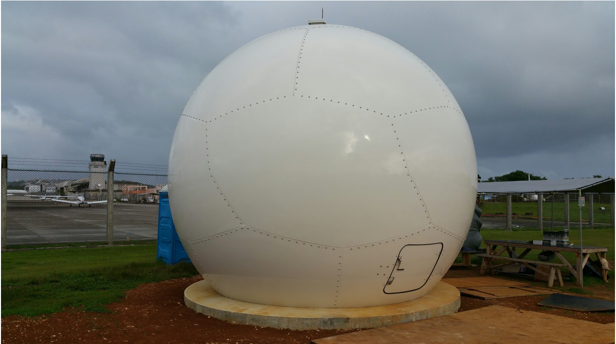
Figure 97. Taken shortly following installation, this photograph shows the radome on the antenna pad. The antenna is inside. The antenna dish is three meters (9.8 feet) wide. The radome is measures approximately 18 feet in diameter, and is capable of withstanding winds up to 190 miles/hour.
