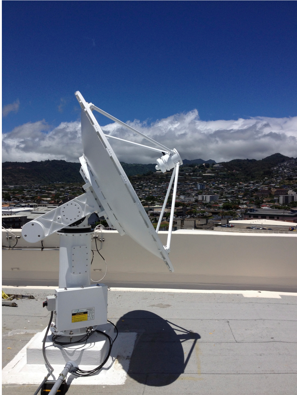
Figure 11.1. X/L-band antenna installed at Honolulu Community College on 8 August 2012.
