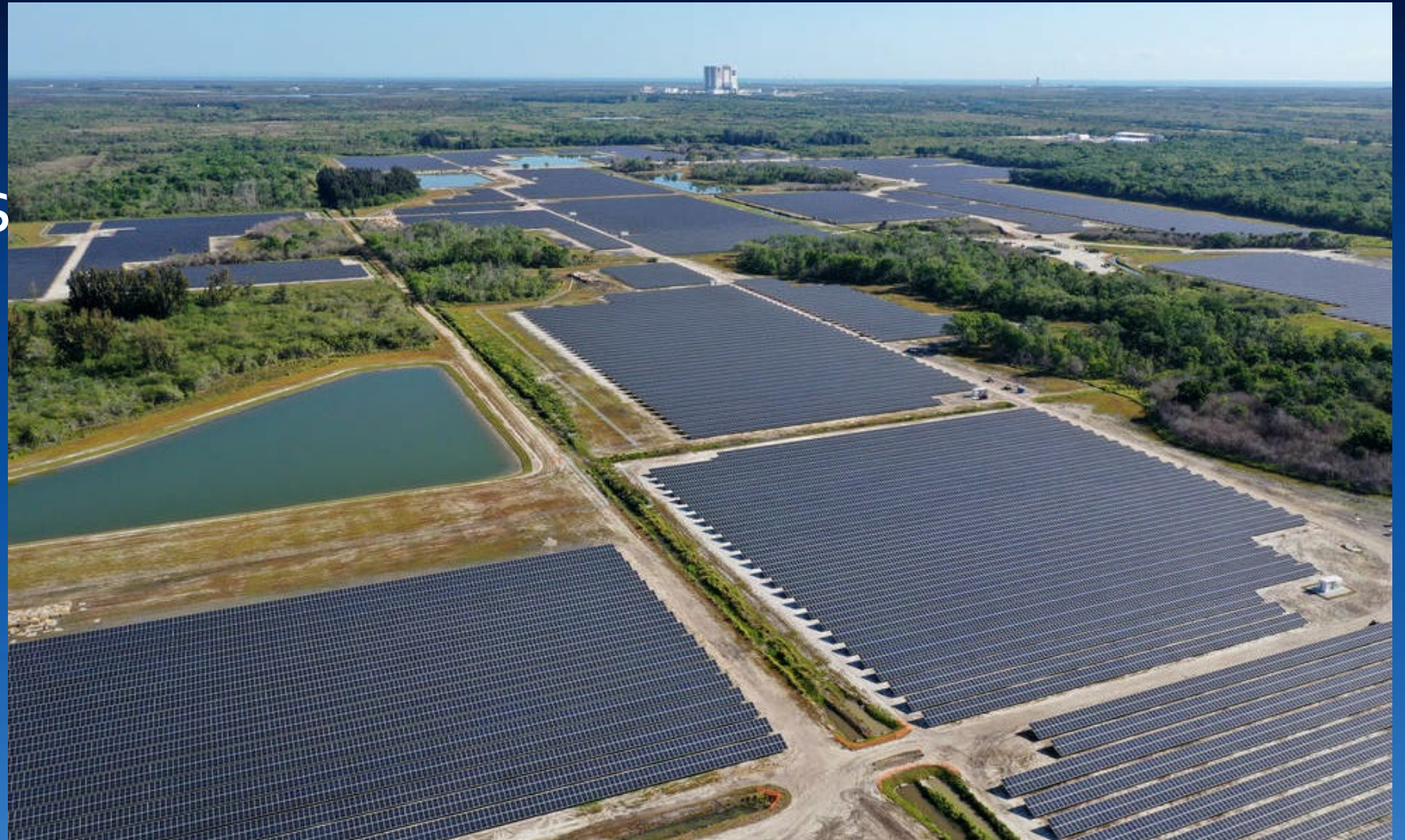
Florida Power and Light's (FPL) 74.5 megawatt solar site, spanning 491 acres at NASA's Kennedy Space Center in Florida.
